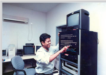
Fixing Editing system (AVID), Cabling & making the Patch Panel in the first "Swarnavahini" studio, Sri Lanka.
